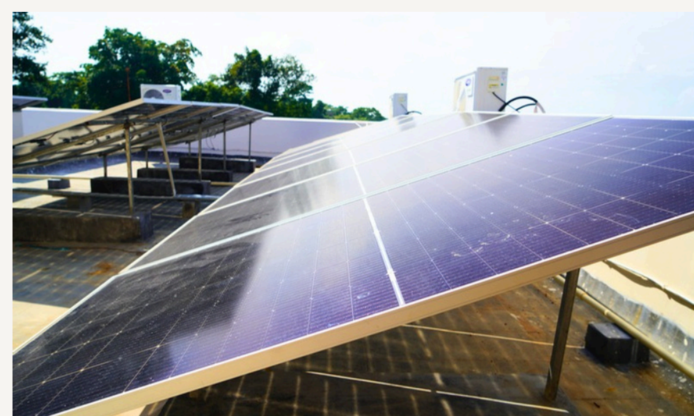
Roof-Top Solar Power Panels at various buildings in the campus
